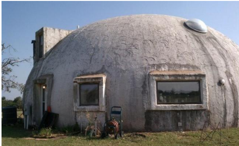
Figure 2.9: A dome hit by a tornado in Blanchard, OK (Josh South)
